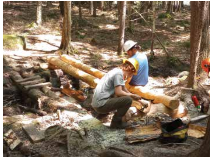
Student volunteers finalize a new log bridge on the Cranberry Meadow Pond Trail in Peterborough
